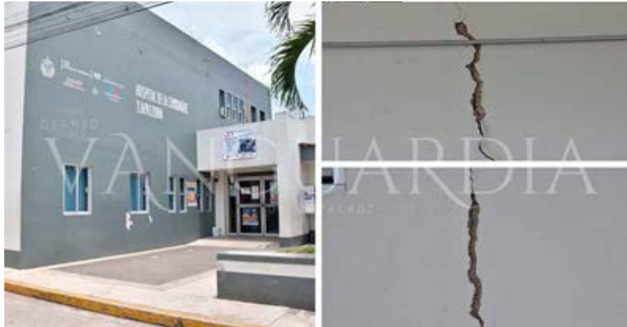
Figure 7.21. Damage to the Civil hospital at Tlapacoyan, Veracruz (Vanguardia, 2020).
