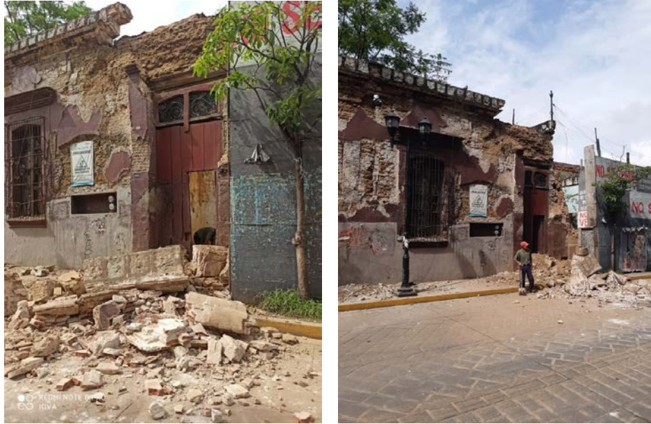
Figure 7.16. Damage to the facade of the historical building located at the center of Oaxaca (Twitter, 2020q; Twitter, 2020i).
