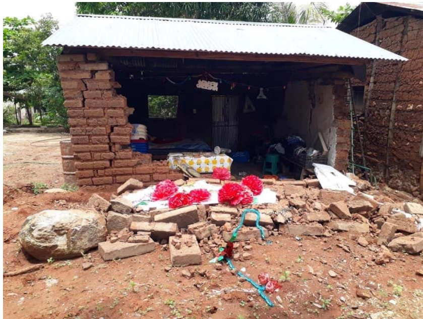
Figure 7.5. Out-of-plane collapse of a wall in an adobe house (Twitter, 2020g).
