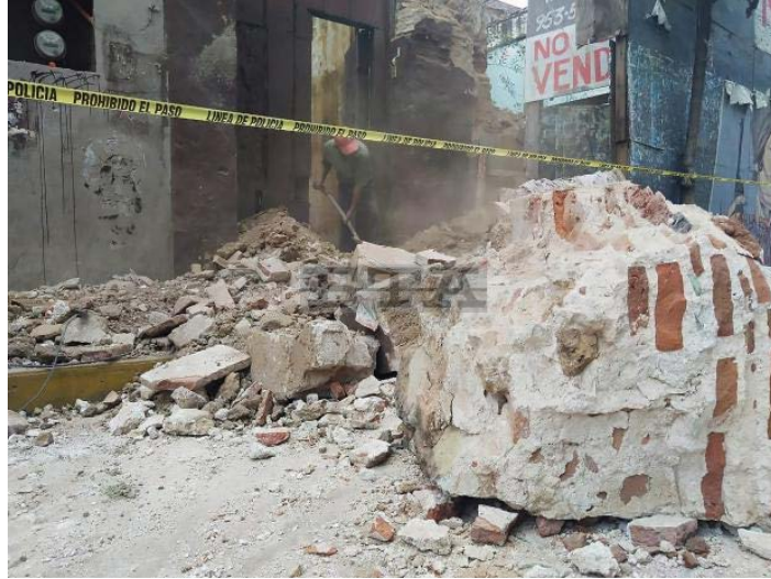
Figure 7.7. Masonry debris after single family building collapse in Oaxaca City (Daily Mail, 2020).
