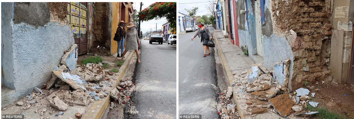
Figure 7.15. Failure of masonry walls and spalling of plaster in Oaxaca (Distinct Today, 2020).
