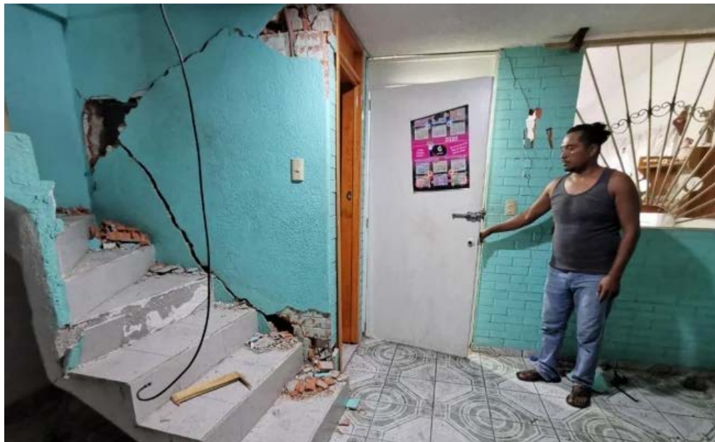
Figure 7.8. Damage to masonry bearing wall in the first story of a two-story residential structure in Oaxaca (El Universal, 2020c).
