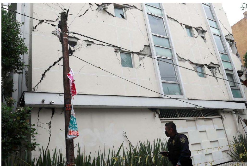
Figure 8.3. Damage in the building located at Tepic 40 in Mexico City after the 2017 earthquake [top] (Cara, 2017) and after the 2020 earthquake [bottom] (Redacción ADN40, 2020).
