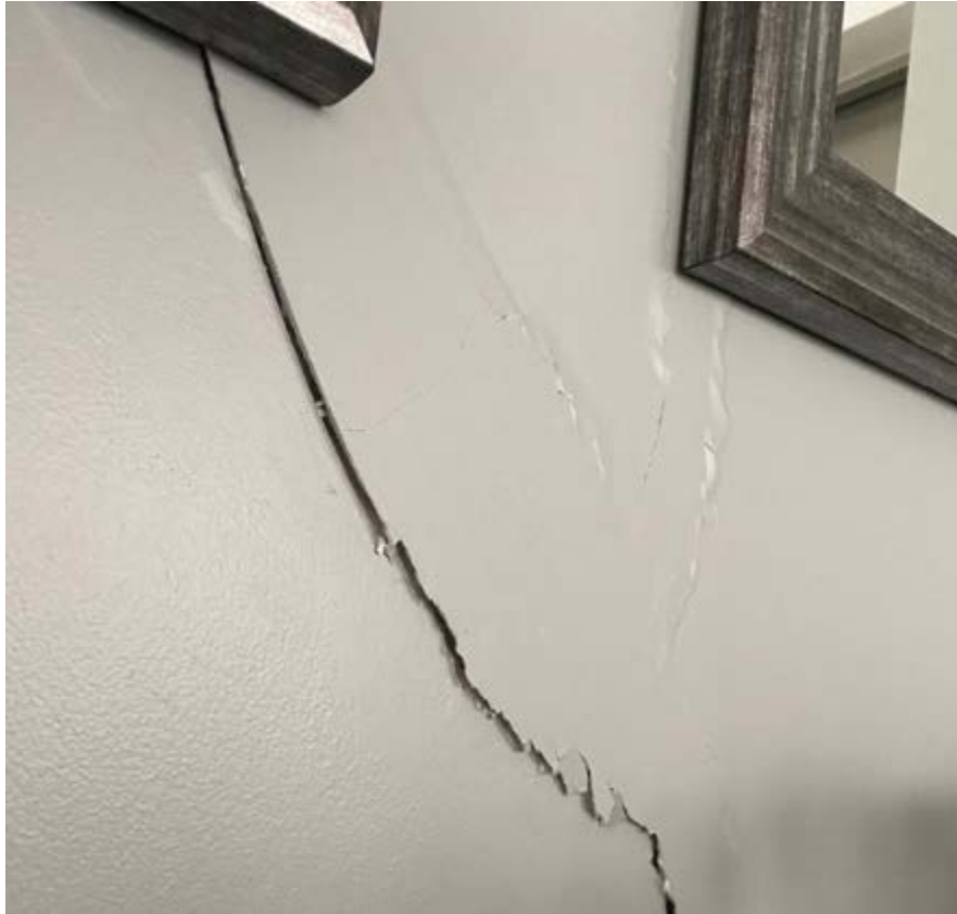
Figure 8.6. Cracking on drywall partition in an apartment building, Mexico City (CNN en Español, 2020).
