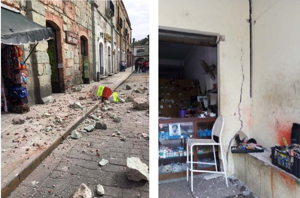
Figure 7.14. Failure of adobe walls in central Oaxaca (left), (Twitter, 2020k) and masonry wing wall damage and detachment (right) (Estado 21, 2020).
