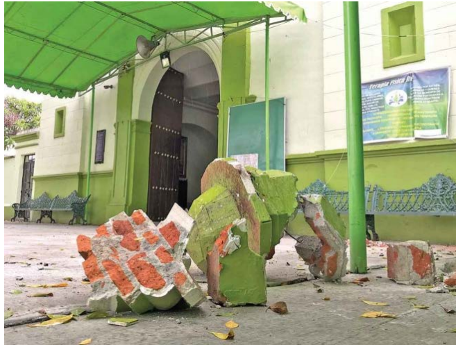
Figure 7.25. Collapse of parapet ornamentation in the church of Santísima Trinidad de las Huertas, City of Oaxaca. (Excelsior, 2020b).
