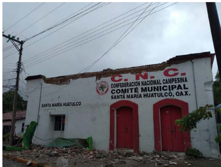
Figure 7.26. Collapsed unreinforced masonry parapet in a government building in Huatulco, Oaxaca (Puerto Vallarta Daily News, 2020).
