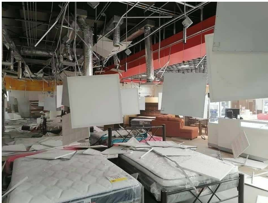
Figure 7.27. Collapsed acoustical ceiling in a furniture store in the city of Oaxaca (Facebook, 2020c).
