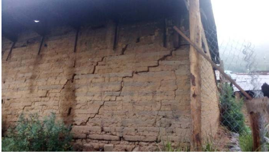
Figure 7.4. Severe diagonal tension cracking in a wall of an adobe house, Oaxaca (Its going down, 2020).
