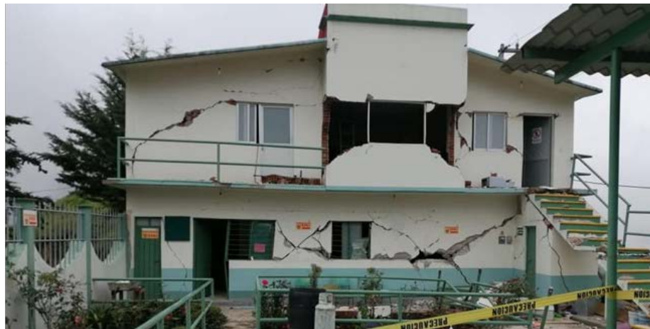
Structural failure of a medical unit located in Oaxaca, Mexico (Twitter, 2020).
