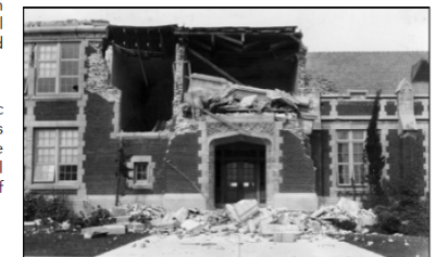
View of John Muir School, showing damage from the March 10, 1933 Long Beach earthquake. Located on Pacific Ave. in Long Beach, California. Photo taken 8 days after, on March 18, 1933. (photo: W.L. Huber, source: USGS, 1993).
