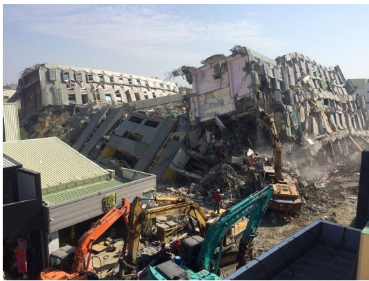
14-story Condominium 2016 Meinong EQ
